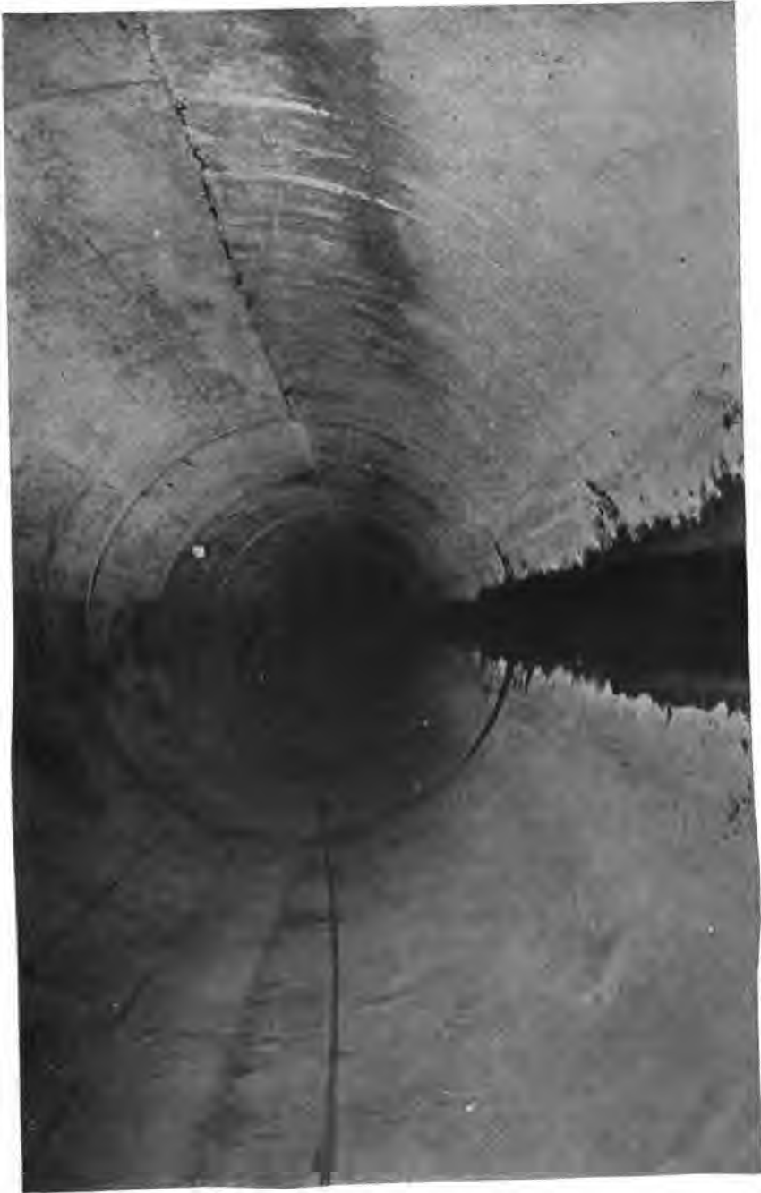
PLATE 108.—Completed Pressure Tunnel Lining. Note smooth finish and close joints at invert and springing line. Concrete surface very dry under high ground water bend.
